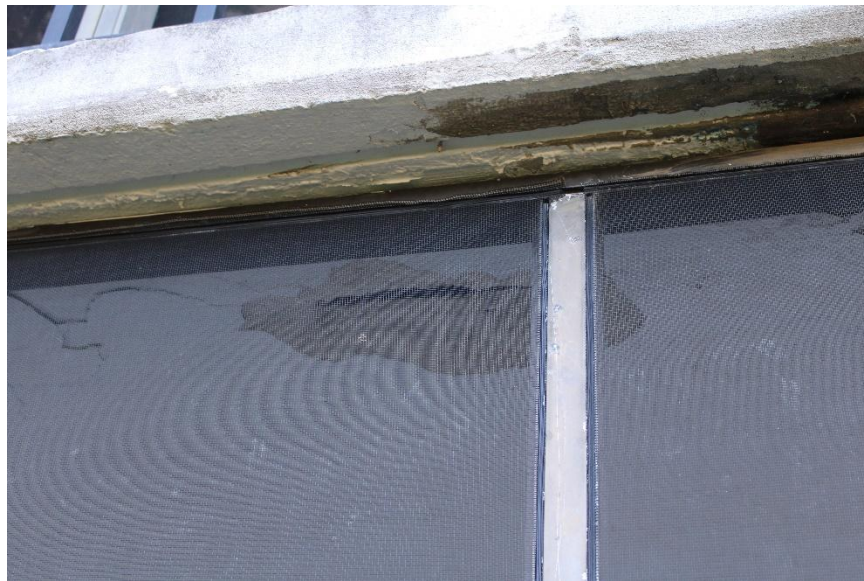
Photograph 4 – View of Overhead Spall.
