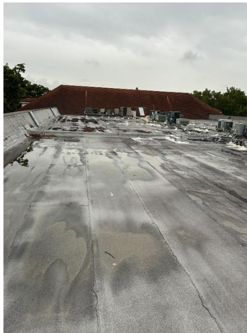
Photograph 8 - Visible cracks, patches, and weathered surfaces on the roof need routine maintenance.
