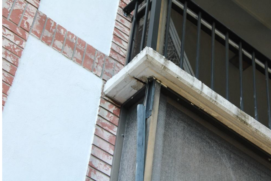
Photograph 7 – Visible Spalding on a balcony.
