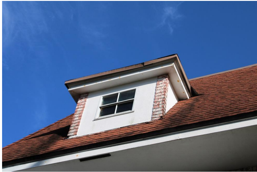
Photograph 3 – View of the building envelope, featuring a window area and above resting on wood trim combined with decorative veneer stone.
