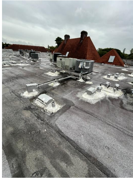
Photograph 5 – Overview of the roof showing the surface, HVAC equipment, and other utilities. Regular maintenance is required to address wear and ensure proper functionality.
