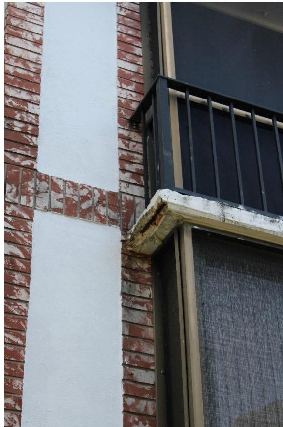
Photograph 6 – Visible Spalding and rebar exposed on the outer edge of the balcony.
