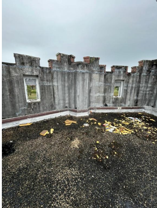
Photograph 7 - Rooftop area with exposed concrete parapets showing signs of weather and scattered debris. Evidence of ongoing maintenance
