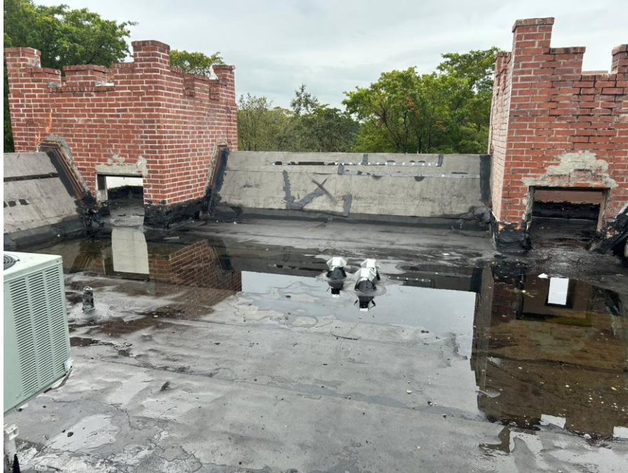
Photograph 5 – View of roof with standing water, patched areas, and exposed concrete. Evidence of drainage issues and recent repair work, possibly to address water infiltration or leaks.
