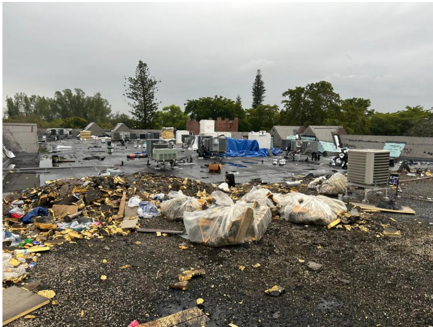
Photograph 6 – View of roof under renovation with construction debris, discarded insulation, and various HVAC units.
