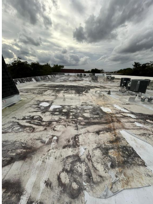
Photograph 5 – View of aged flat roof with deteriorated and discolored membrane, showing signs of wear, peeling, and previous patchwork.
