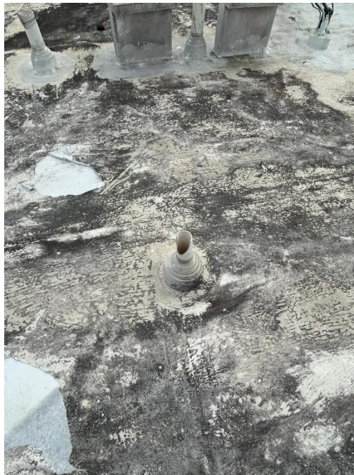
Photograph 6 -View of vent pipes and deteriorated membrane showing discoloration, patchwork, and signs of aging. Sealant has been applied around penetration, indicating efforts to manage leaks or water infiltration.
