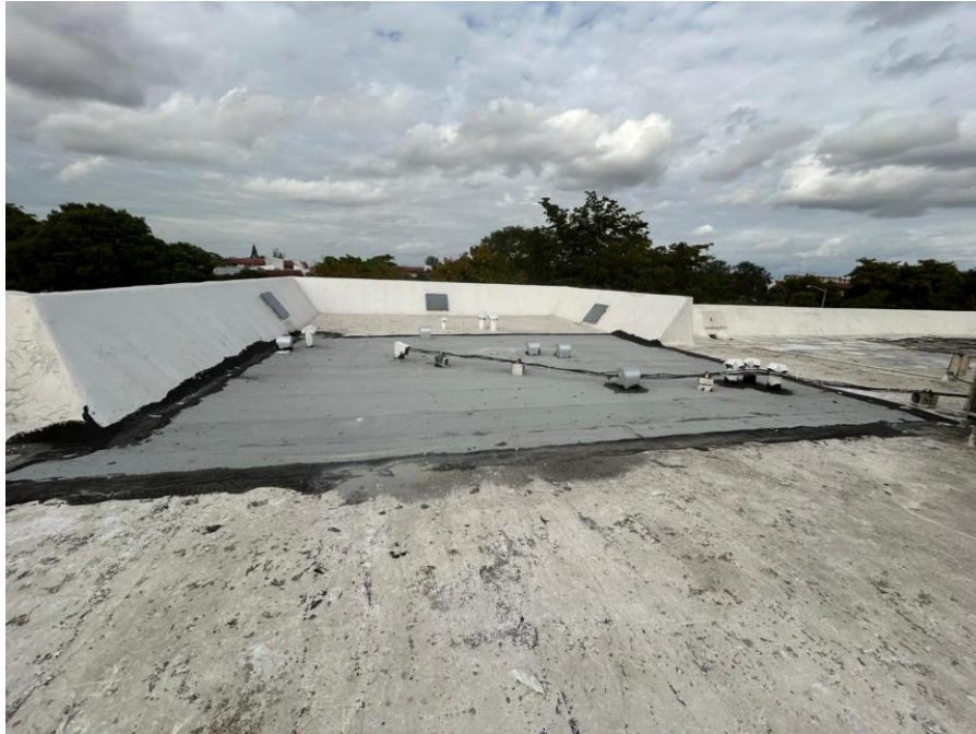
Photograph 7 – View of roof with coated parapet walls and a repaired membrane section secured with waterproofing sealant.
