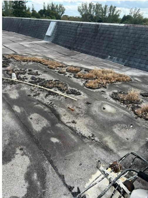
Photograph 5 – View of roof with overgrown vegetation, deteriorated membrane, and visible signs of neglect.
