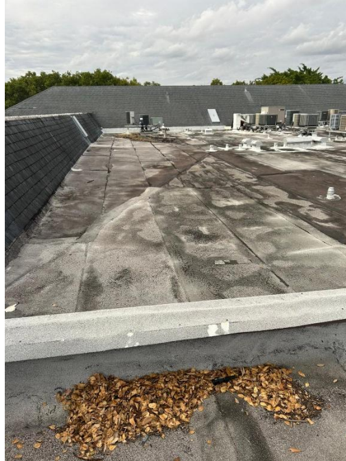
Photograph 7 - Mansard roof with shingle cladding and a flat central section showing signs of wear, discoloration, and previous repairs. Accumulation of leaves and debris suggests potential drainage issues
