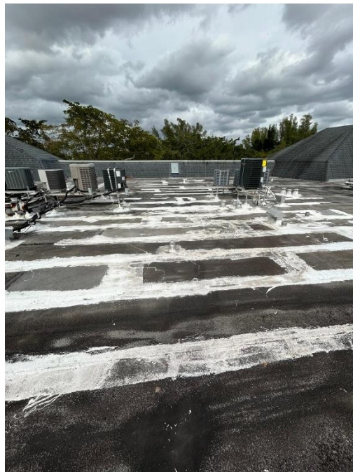
Photograph 6 – View of multiple HVAC units and extensive patchwork, featuring white sealant applied to seams and cracks. The membrane shows signs of aging and previous repairs, suggesting ongoing maintenance.
