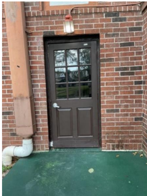
Photograph 14 – typical door, insufficient protection and improperly sealed
