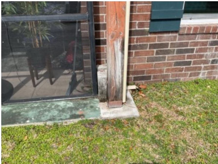
Photograph 6 -- Visible growth of vegetation on the outer edge of the balcony.
