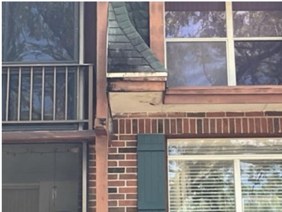
Photograph 2 - View of the balconies and lower roof system, signs of exposure to water and possible sign of mold.
