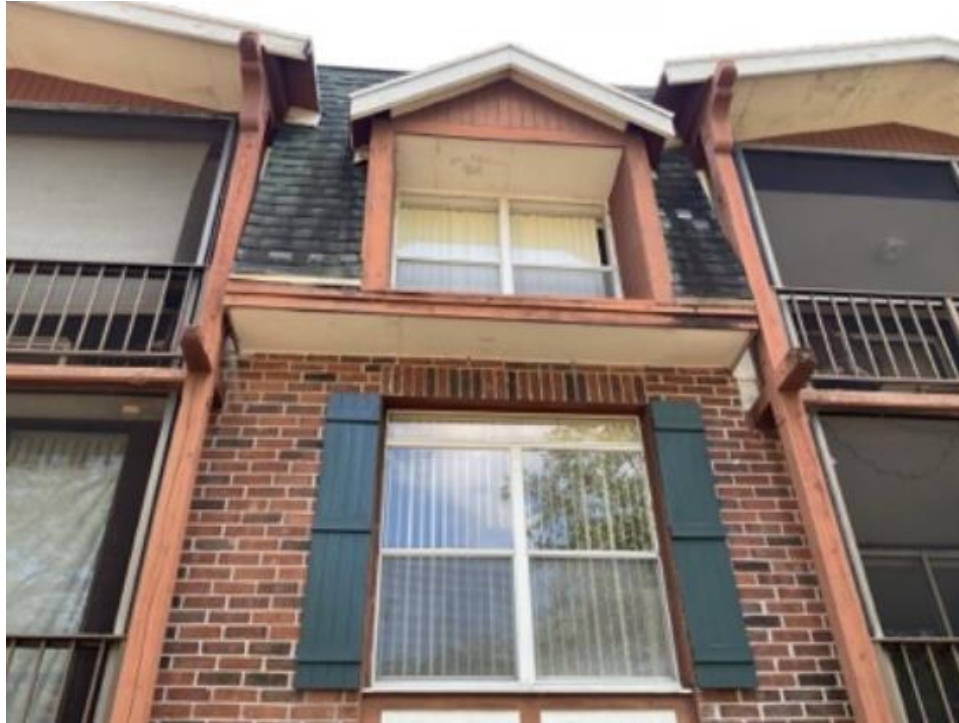
Photograph 3 – View of underside of soffit, sign of water damage.
