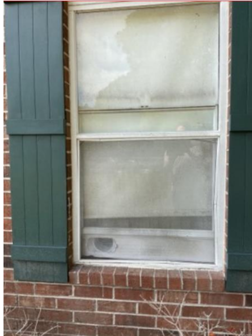
Photograph 13- typical window, insufficient protection and improperly sealed.
