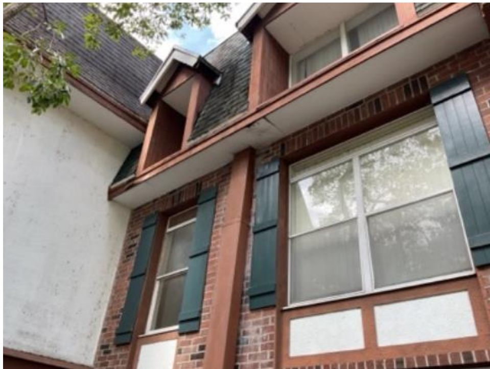
Photograph 4 – Overview of the underside of roof showing the soffit, signs of water damage.
