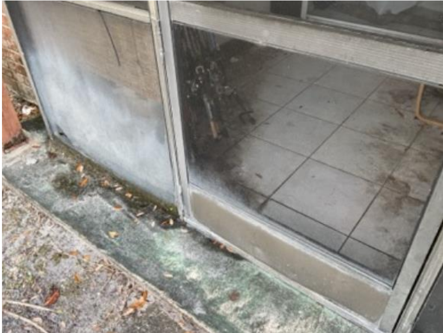
Photograph 7 - Visible growth of vegetation, pooling water, and source of water damage.
