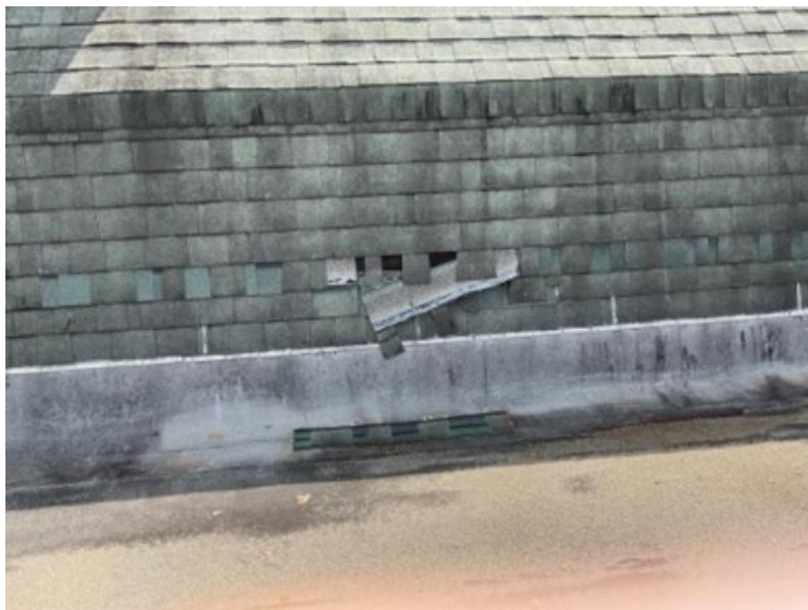
Photograph 12 compromised mansard parapet roof.
