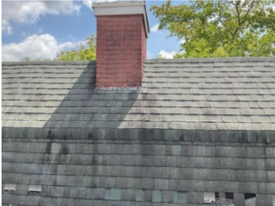
Photograph 11 – compromised mansard parapet roof.
