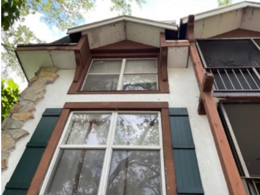
Photograph 5 - Overview of the underside of roof showing the soffit, signs of water damage.
