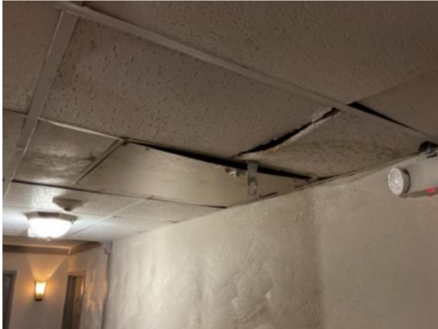
Photograph 9 - View of suspended ceiling on 3 rd floor corridor with evidence of previous water damage.
