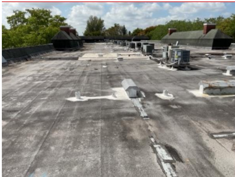
Photograph 10 – View of roof repair with multiple patches and sealant applications, showing areas of asphalt-based waterproofing membrane and white sealant, likely addressing previous leaks or cracks.
