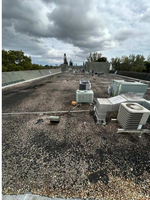
Photograph 5 – Overview of the roof showing gravel surface, HVAC equipment, and other utilities. Regular maintenance is required to address wear and ensure proper functionality.
