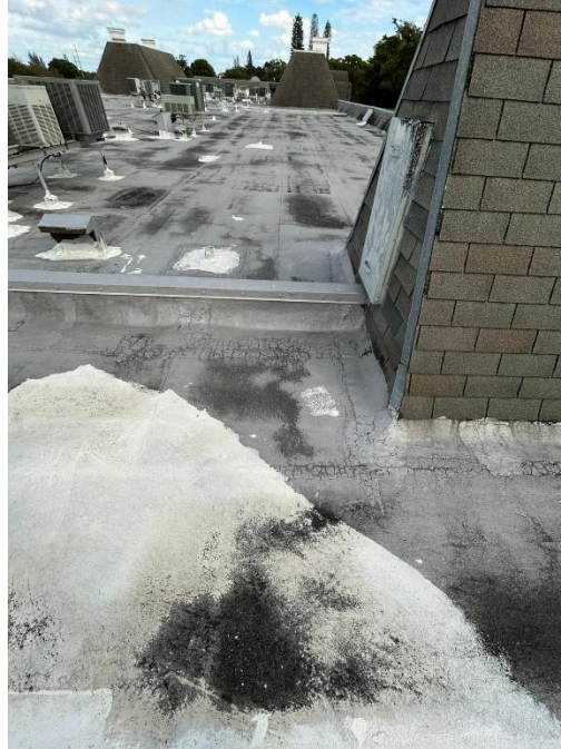
Photograph 5 - Overview of the roof showing visible wear, patching and discoloration, around HVAC units and vent penetrations
