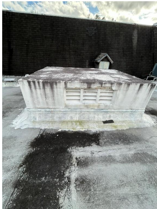
Photograph 8 - Weathered rooftop ventilation structure with visible discoloration, cracks, and patching on the surrounding flat roof surface
