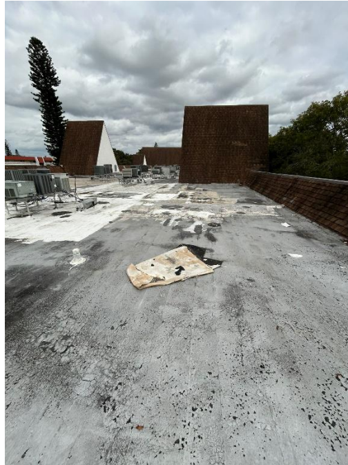
Photograph 5 - Overview of the roof showing Aged coatings and scattered debris.
