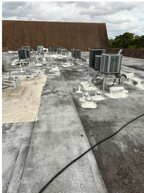
Photograph 6 - Multiple HVAC units, vents, and utility installations, showing signs of weathering, patch repairs, and varying roofing materials.
