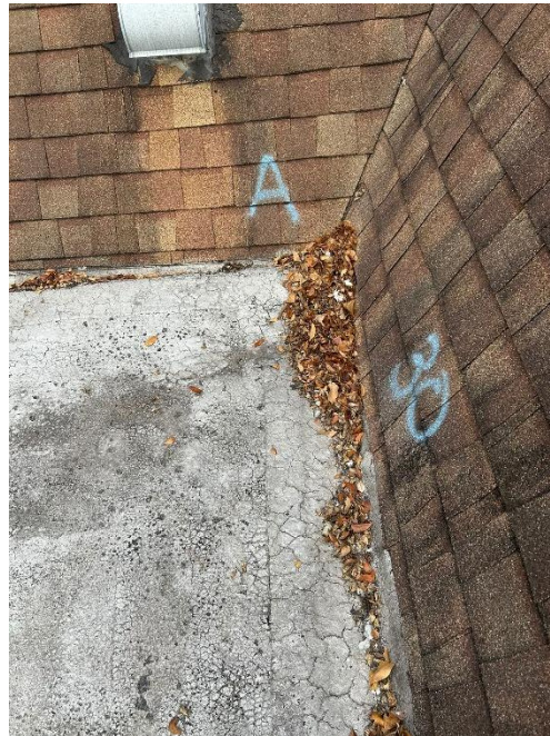
Photograph 8 - Visible cracks, patches, and weathered surfaces. Adjacent sloped shingle roofing shows signs of wear, with debris accumulation along the edge.
