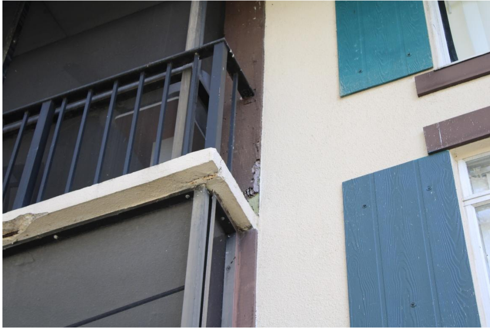
Photograph 3 – View of balcony edge spalling with exposed rebar.
