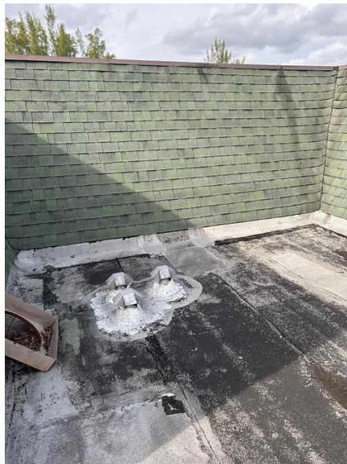
Photograph 8 - Mansard roof with green asphalt shingles showing discoloration and signs of aging, highlighting potential moisture retention and the need for maintenance at the transition to the flat roof.
