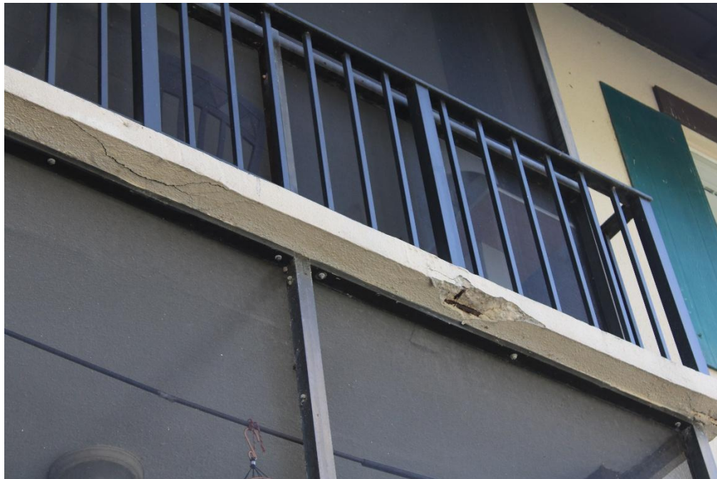
Photograph 6 – View of balcony edge spall with exposed rebar.
